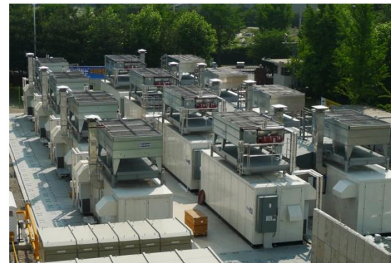
Multi-Megawatt Sites (GS Power, Anyang, South Korea)
